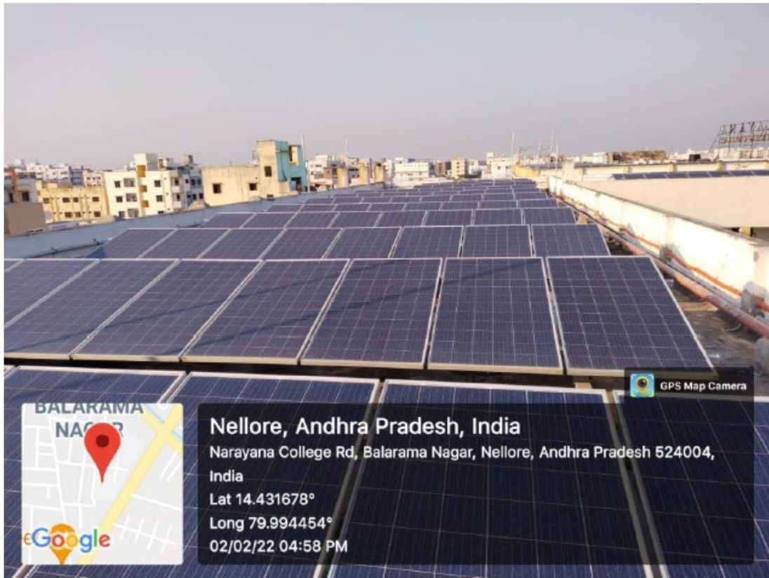
Roof Top Solar Power Plant at Charles Babbage Block
