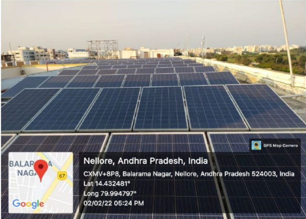
Roof Top Solar Power Plant at Faraday's Block
